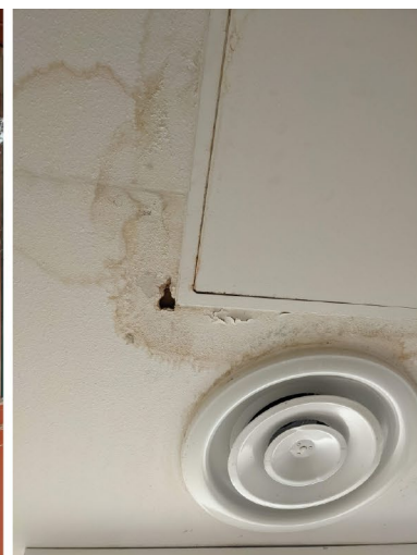
Ceiling water damage due to broken heating, ventilation, and air conditioning system
