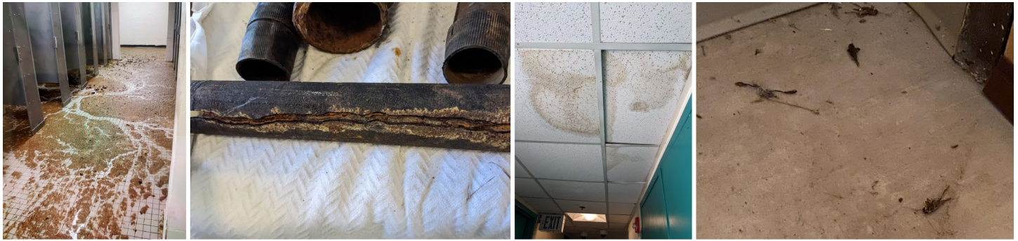
Sewage overflow in training barracks restroom
