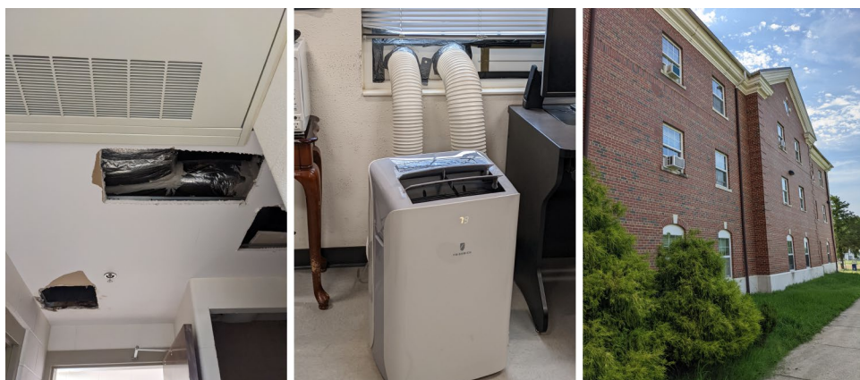
Figure 4: Broken and Supplemental Air Conditioning Systems
