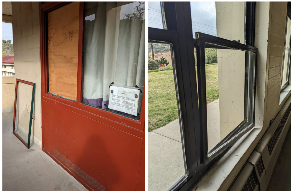
Figure 10: Broken Windows Observed during GAO Site Visits
